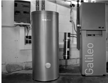
The award-winning fuel cell based combined heat and power unit Galileo 1000 N from Hexis, installed in the basement boiler room of an apartment building.
